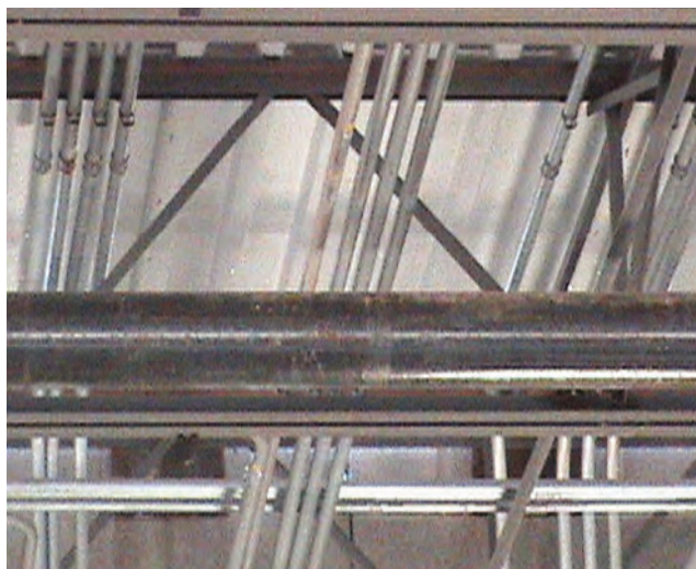
Baker Brother’s realized a projected 20% savings in materials and installation costs on this large job for a mid-west “big box” retailer, and plans to start using 20’ length EMT in many future jobs when applicable.
